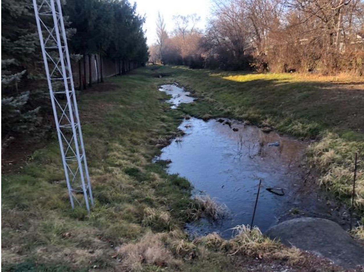
Western portion of storm ditch. In very disrepair and water sits versus being conveyed.
