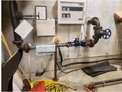
Domestic Water Service
