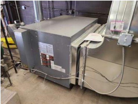
Ducted Gas-Fired Unit Heater
