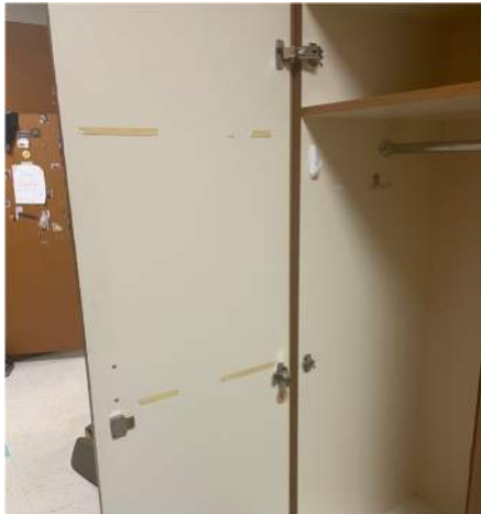
Failing Locker Unit at Men's
