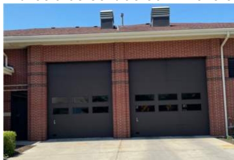
Apparatus Bay Overhead Doors
