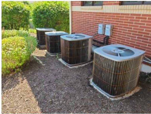
Air-cooled Condensing Units (typ. 4)
