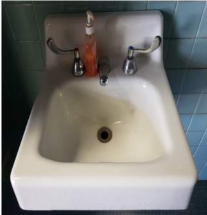
Sink at Apparatus Bay Toilet
