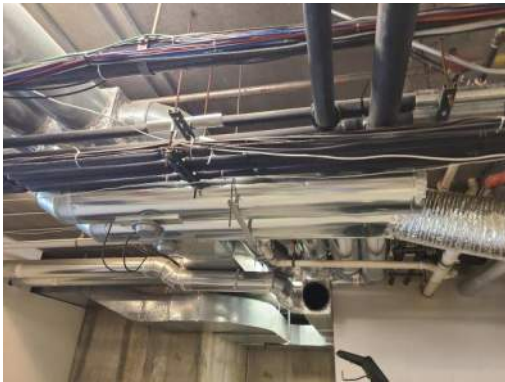
Open-ended Basement Ductwork
