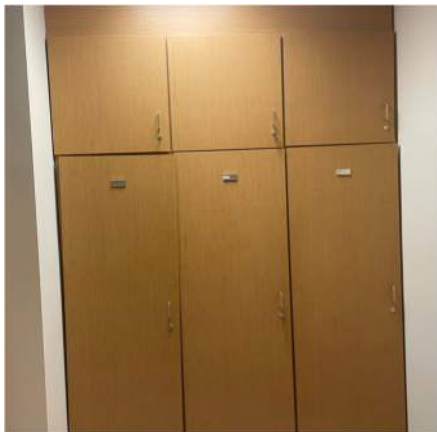
Failing Locker Unit at Women's
