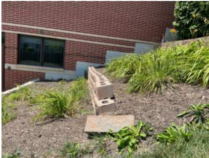
Failing Retaining Wall
