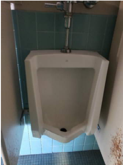
Urinal at Apparatus Bay Toilet
