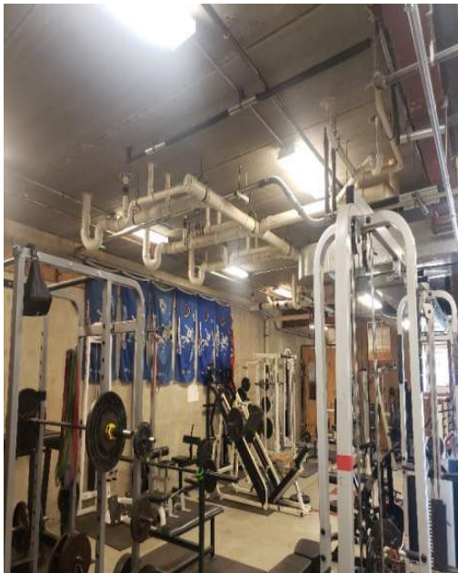
Exposed Piping at Lower Level
