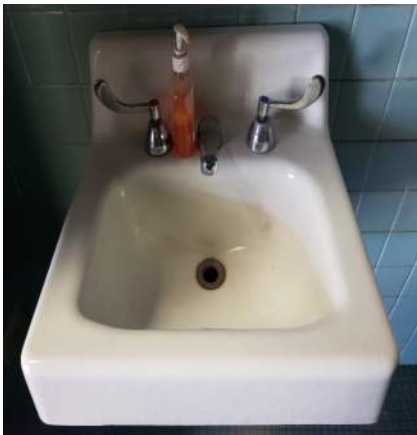
Sink at Apparatus Bay Toilet
