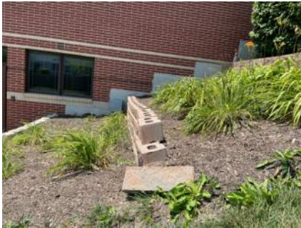
Failing Retaining Wall
