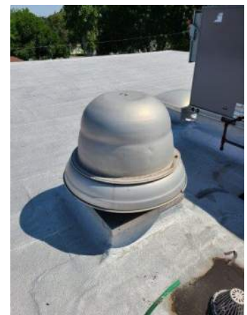
Roof Mounted Exhaust (typ.)
