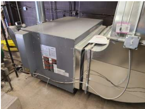
Ducted Gas-Fired Unit Heater
