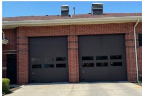
Apparatus Bay Overhead Doors
