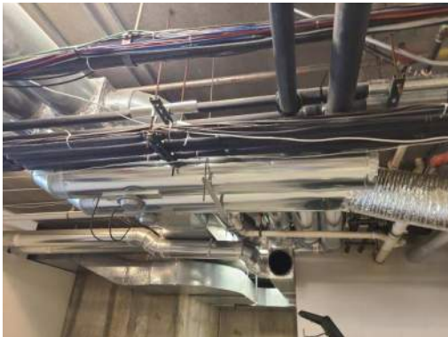
Open-ended Basement Ductwork
