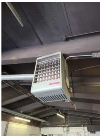
Gas-fired Unit Heater
