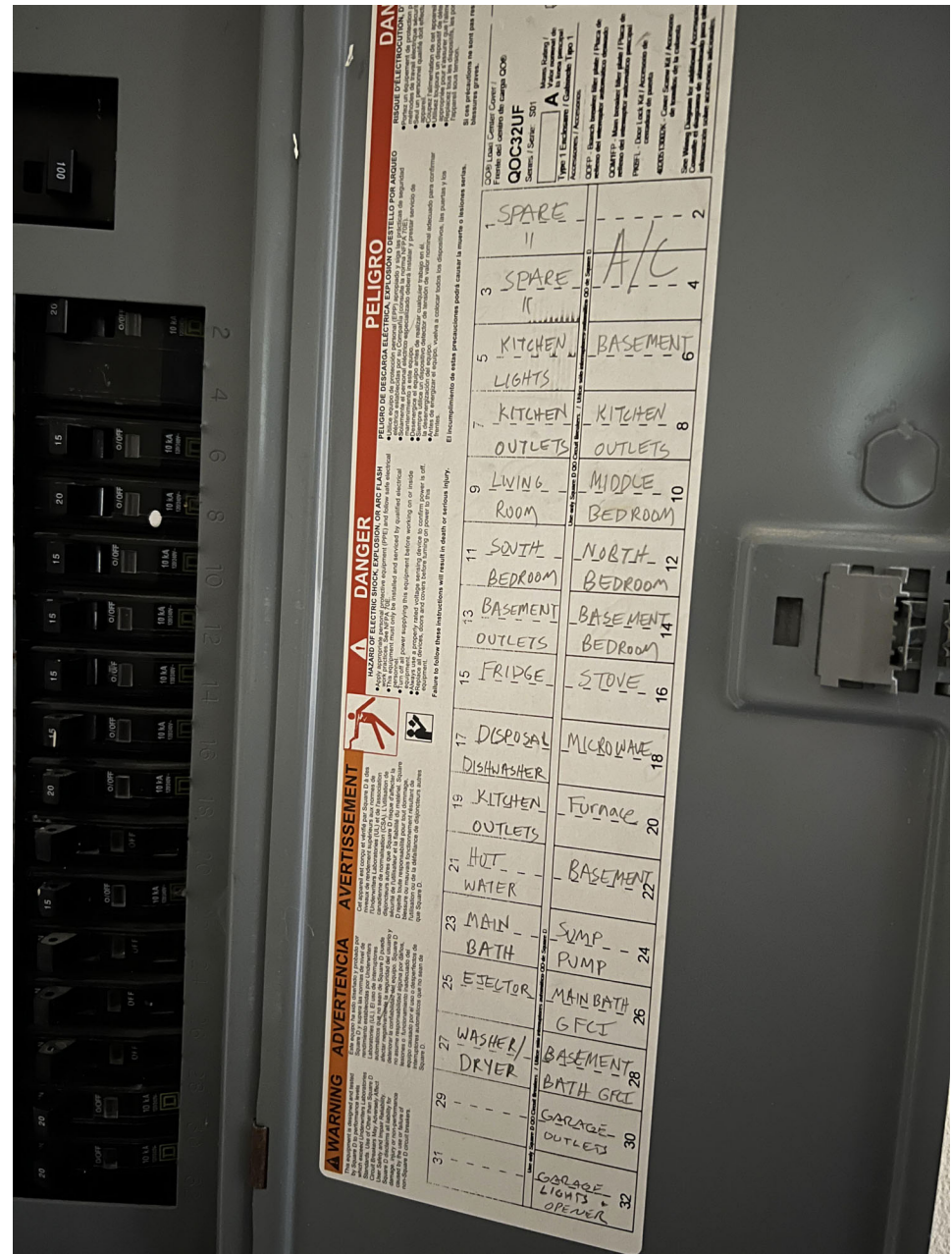
EXISTING 100 AMP ELECTRICAL PANEL
