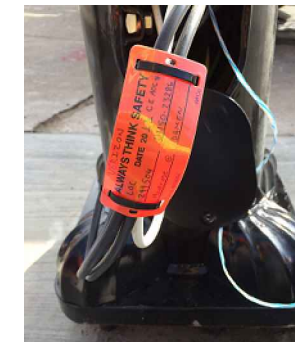
SAMPLE TAGGING IN POLE HANDHOLE
